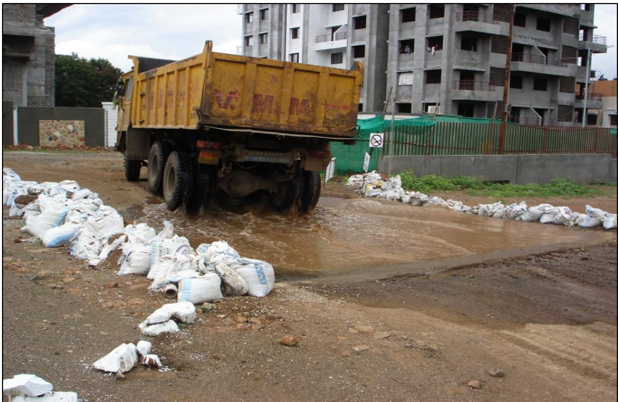
Picture No. 3-2: Water pit at entry and exit points for washing of truck tyres
