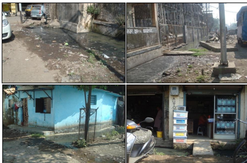
Picture No. 2-39: Open sewage drains in Kalyan Dombivali area
