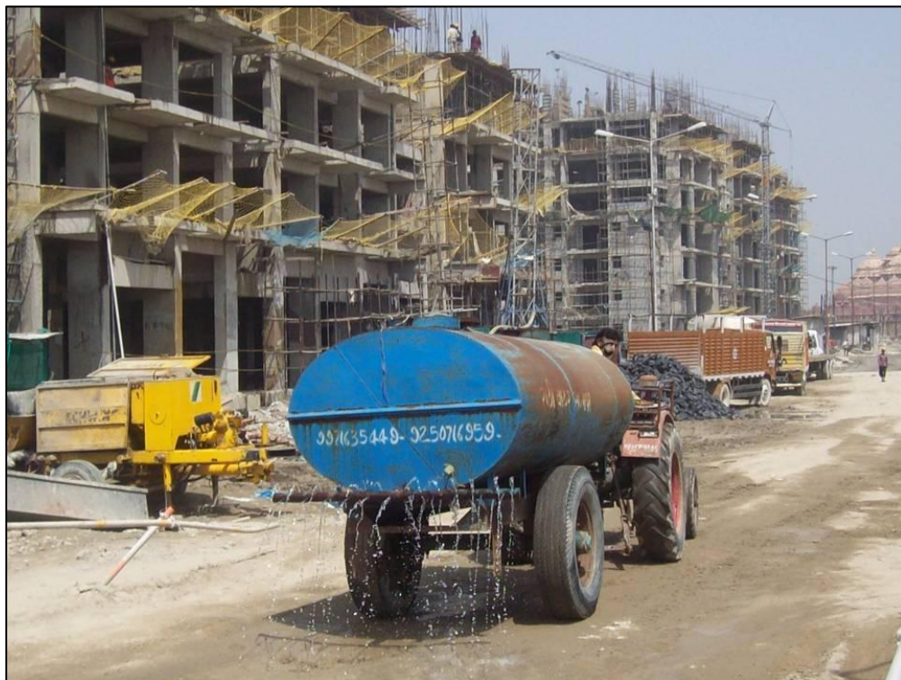
Picture No. 3-3: Sprinkling of water to reduce dispersion of dust at the construction site
