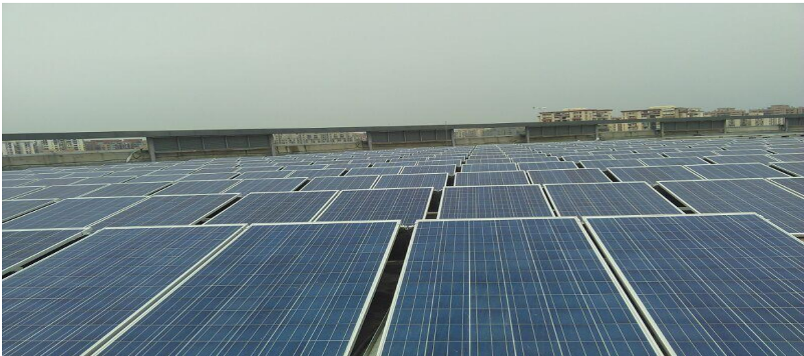
Solar PV Power panel
