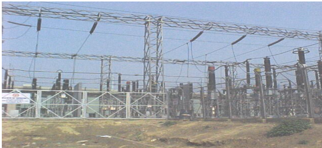
Typical High Voltage Receiving Sub-station
