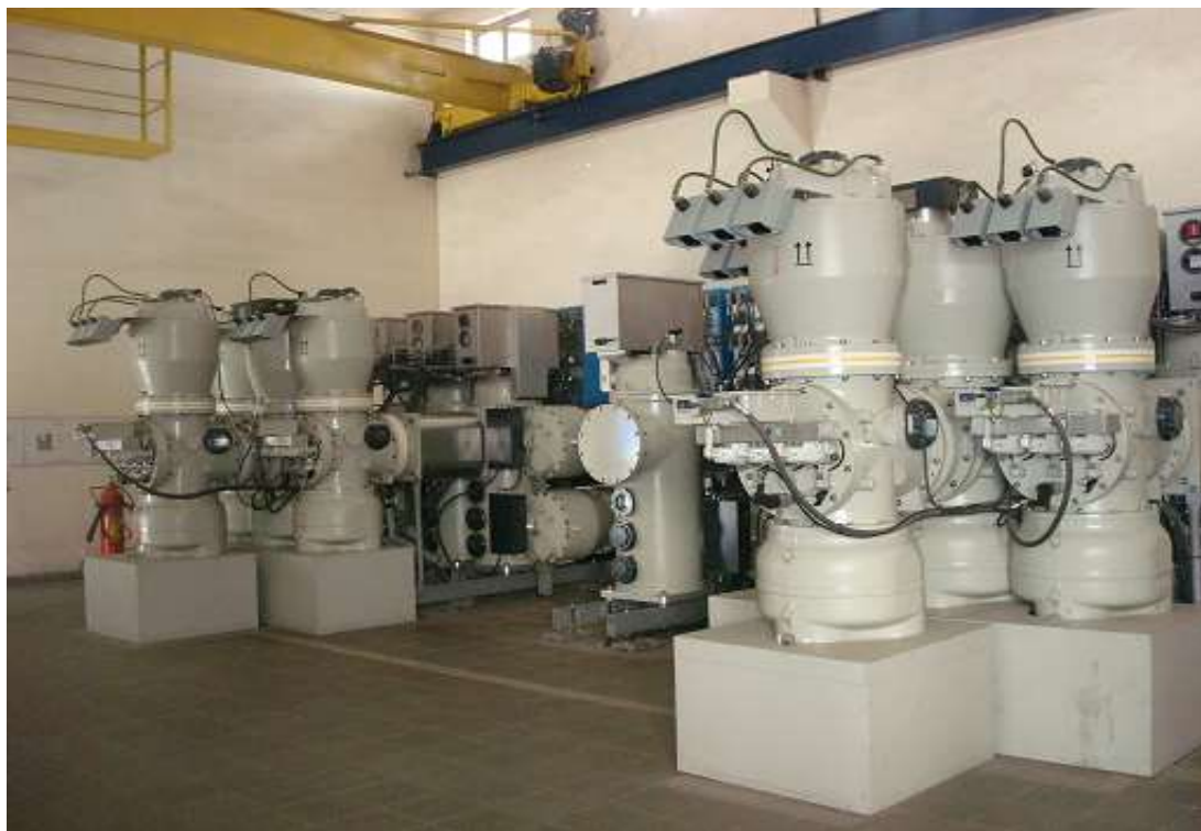
Typical High Voltage Gas Insulated Sub-Station (GIS)
