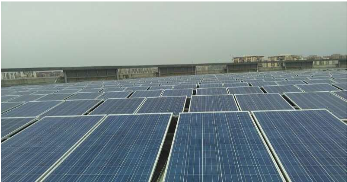
Solar PV Power panel
