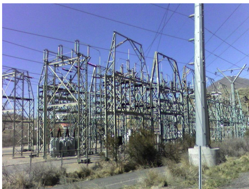
Figure 11.1: Typical Receiving Sub Station
