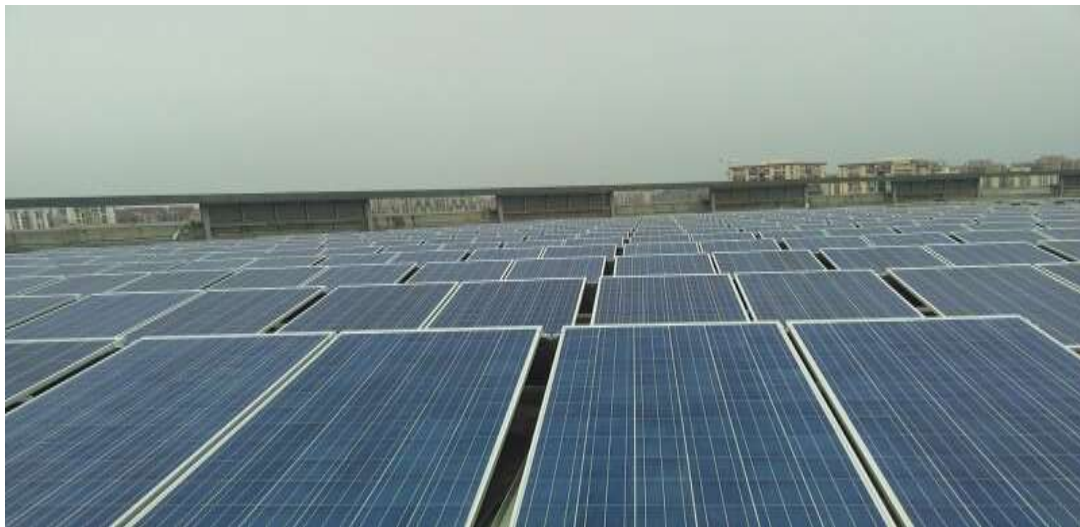
Solar PV Power panel
