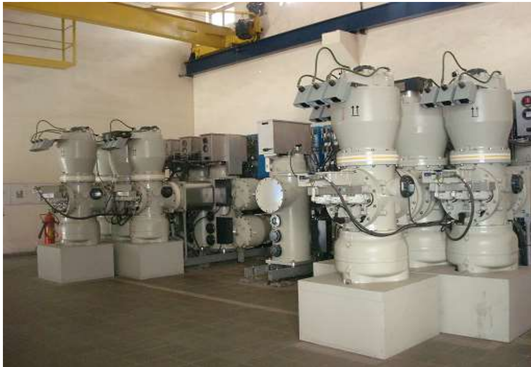
Typical High Voltage Gas Insulated Sub-Station (GIS)
