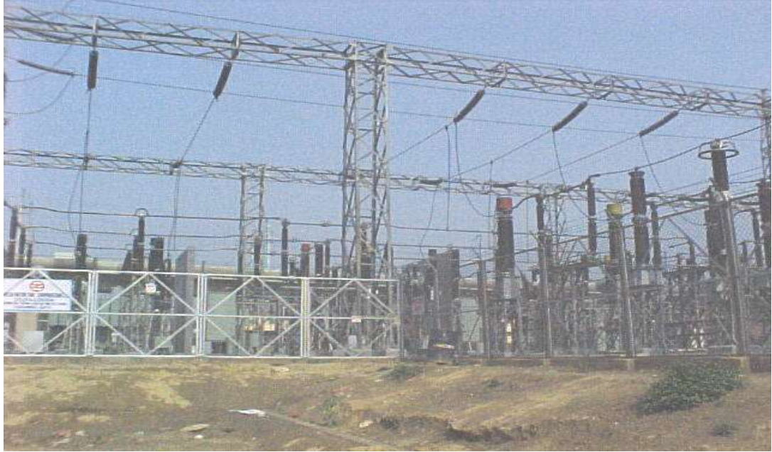
Typical High Voltage Receiving Sub-station
