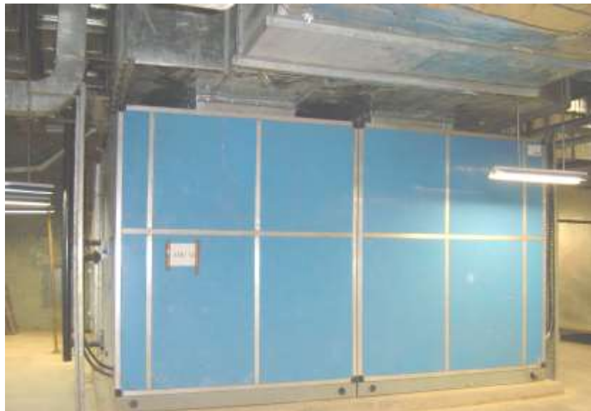
Air Handling Unit
