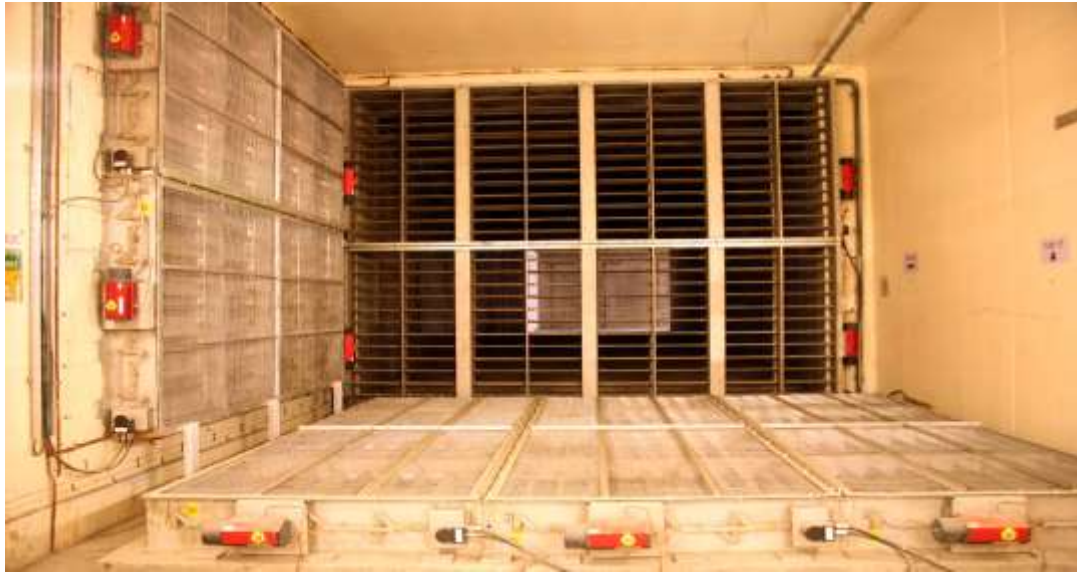
Tunnel Ventilation Dampers
