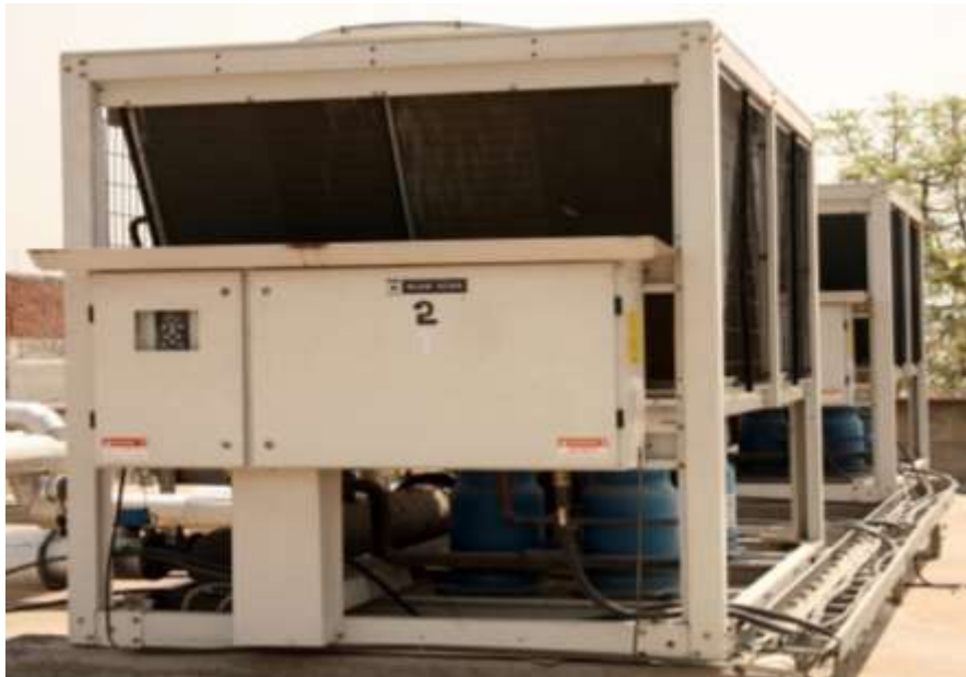
Air Cooled Chiller
