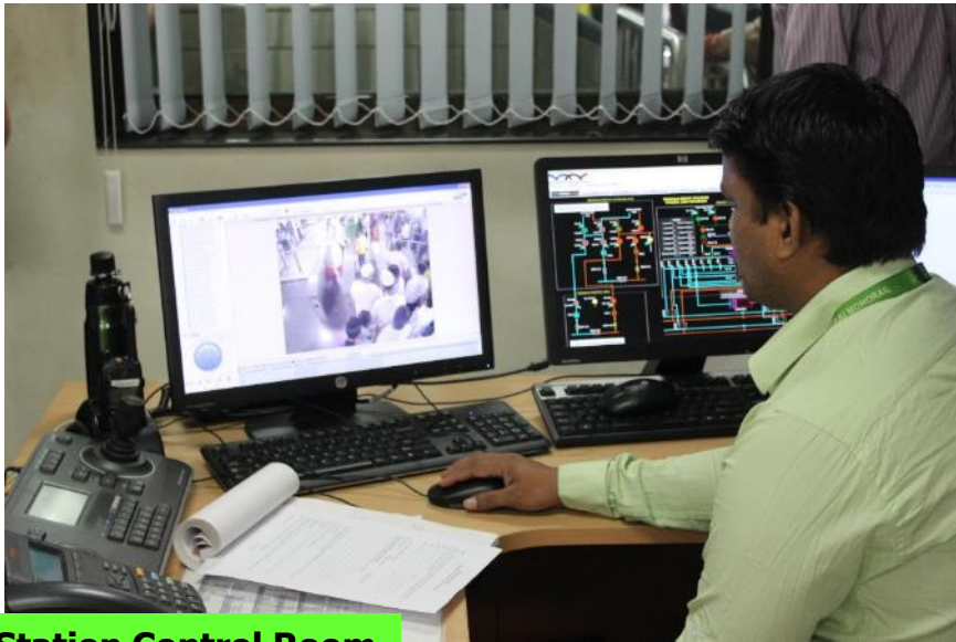
Station Control Room
