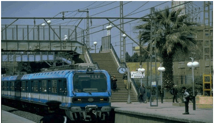
Catenary / 3 rd rail
